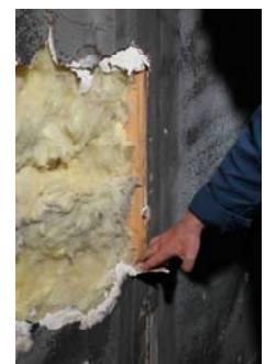
Burned plasterboard is ripped away to show no damage to the timber frame structure at all
